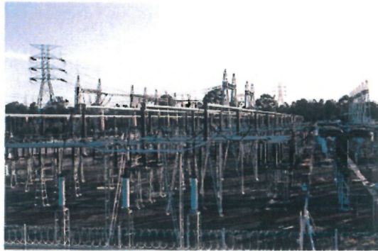
THE 1KM SQUARE SUB STATION IN THE RURAL COUNTRYSIDE NEXT TO SETTLEMENTS
